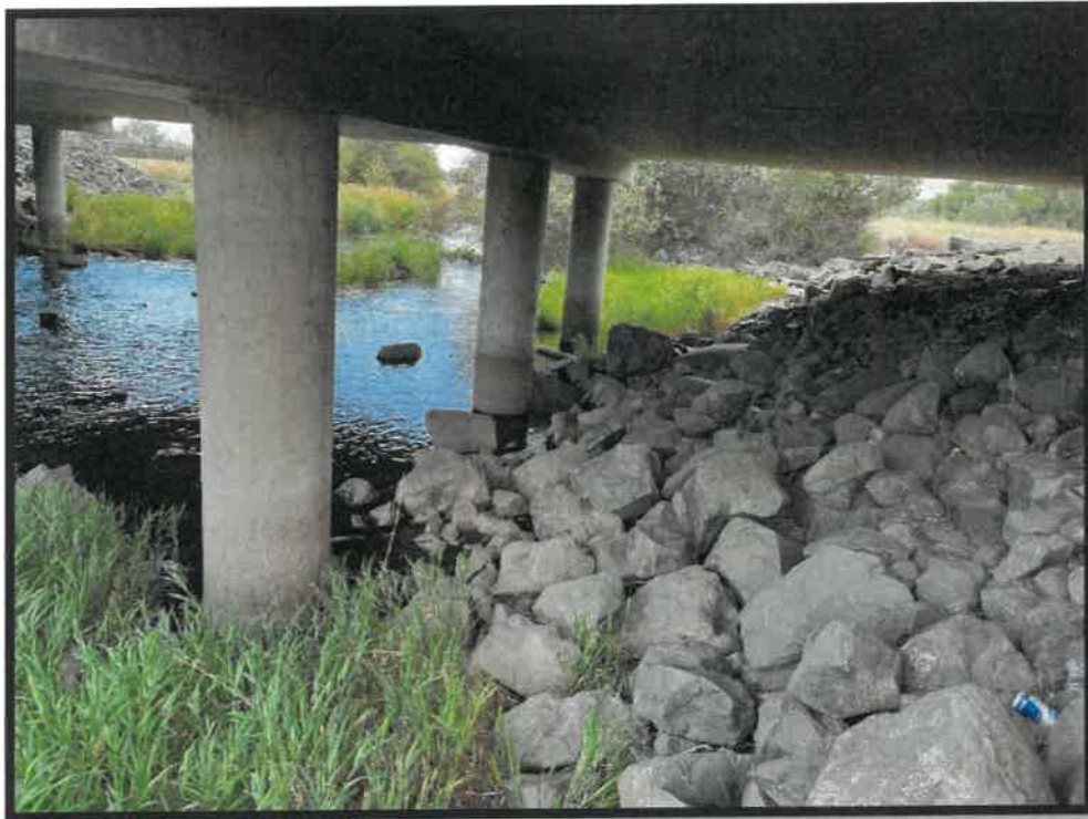
Figure 1: Rip rap beneath EB Wilson Creek bridge. Note submerged pier columns and OHHM.
