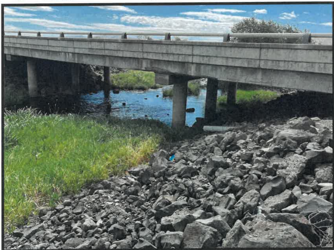
Figure 2: View of EB Wilson Creek facing southwest. Note soffit spalling to be repaired.
